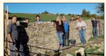
The walling gang take a welcome break in the sun and show off the results of their work
